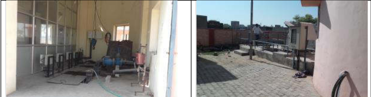
Existing SPS at Kharia Talab
