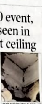
Cracks seen in the ceiling of the Agra Fort after the G20 event. ASI officials refused to comment on the cracks seen in the ceiling of the Agra Fort after the G20 event.
